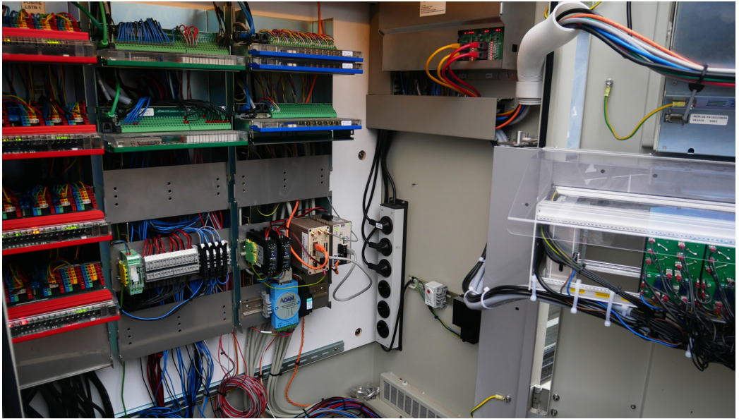
One of the upgraded cabinets containing the equipment that controls the traffic signals at a busy intersection in central Amsterdam. A Wolverine Ethernet Extender connects the cabinet to the traffic signals via an existing copper cable and an MRD 4G router connects the intersection to the control room over the mobile network.
